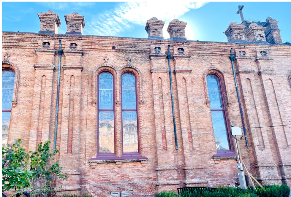
PHASE I - EXTERIOR Renovations (Constance St. side is complete! (picture taken: Dec. 5, 2024)
