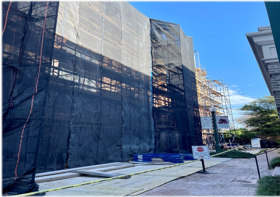
PHASE I - EXTERIOR Renovations are underway (on the riverside of the Church) (picture taken: Dec. 14, 2024)
